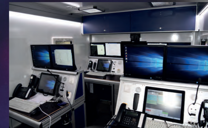
Radio room MCU 2
